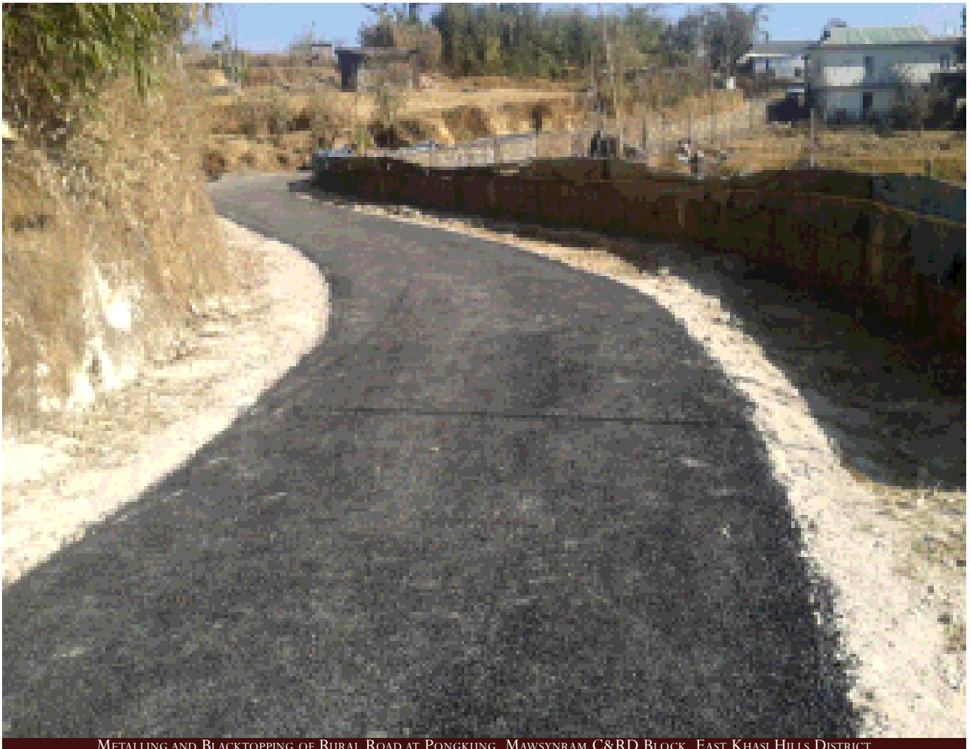
METALLING AND BLACKTOPPING OF RURAL ROAD AT PONGKUNG, MAWSYNRAM C&RD BLOCK, EAST KHASI HILLS DISTRICT
