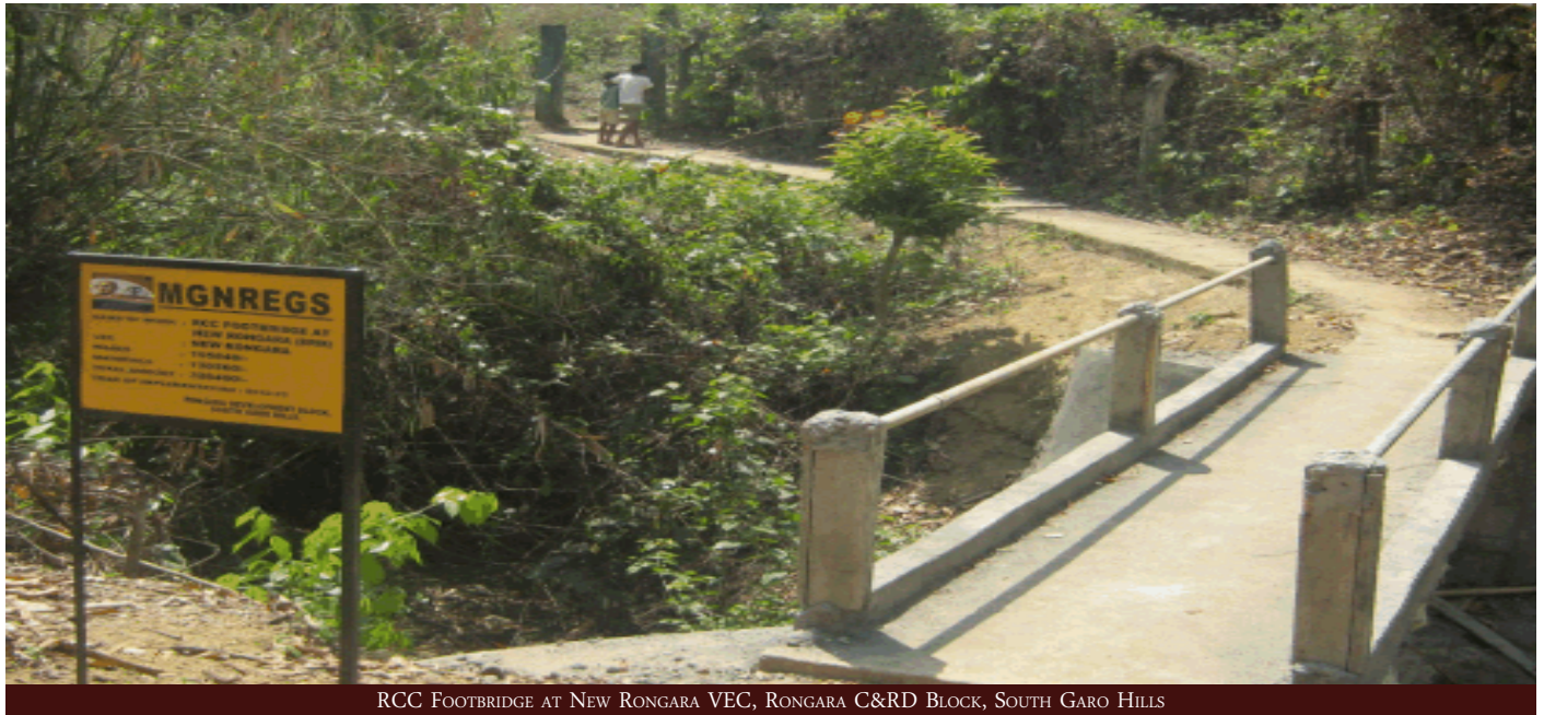
RCC FOOTBRIDGE AT NEW RONGARA VEC, RONGARA C&RD BLOCK, SOUTH GARO HILLS
