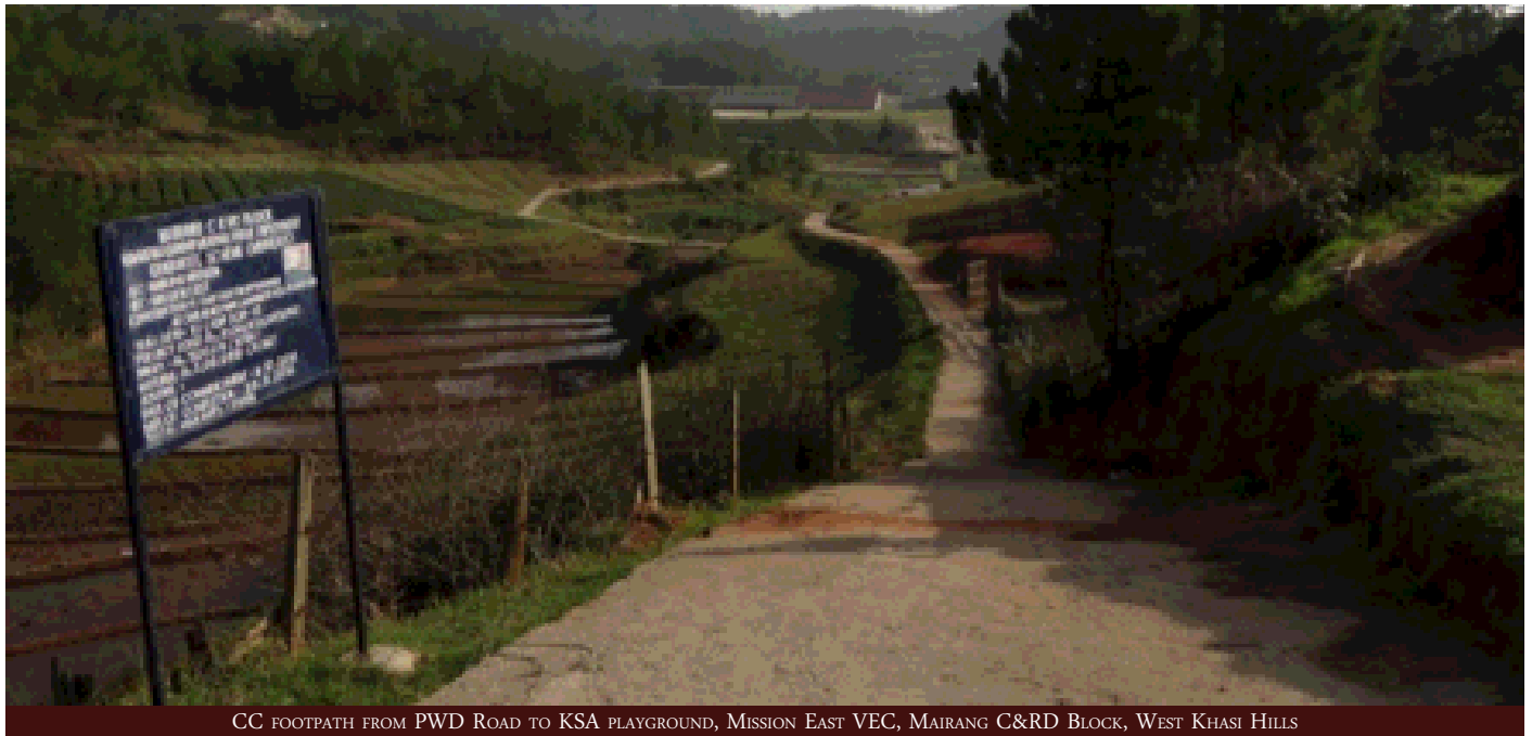
CC FOOTPATH FROM PWD ROAD TO KSA PLAYGROUND, MISSION EAST VEC, MAIRANG C&RD BLOCK, WEST KHASI HILLS
