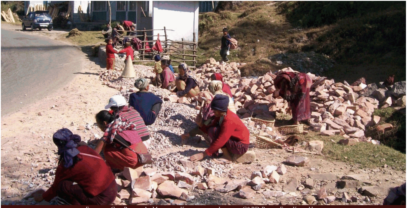
FOOTPATH CUM RAILING AT MAWKDOK, KHATARSHNONG LAITKROH C&RD BLOCK, EAST KHASI HILLS
