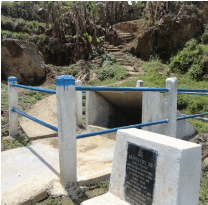
CONSTRUCTION OF DRINKING WATER WELL AT MAWKATAD VEC, MAWTHADRAISHAN C&RD BLOCK, WEST KHASI HILLS
