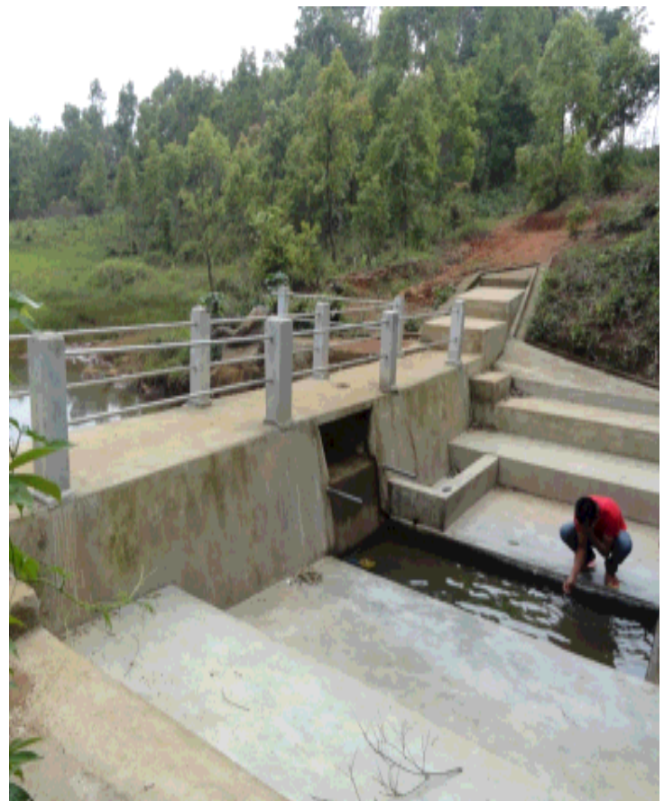
CONSTRUCTION OF WASHING PLATFORM AT POMDKHAR VEC, MAWSHYNRUT C&RD BLOCK, WEST KHASI HILLS
