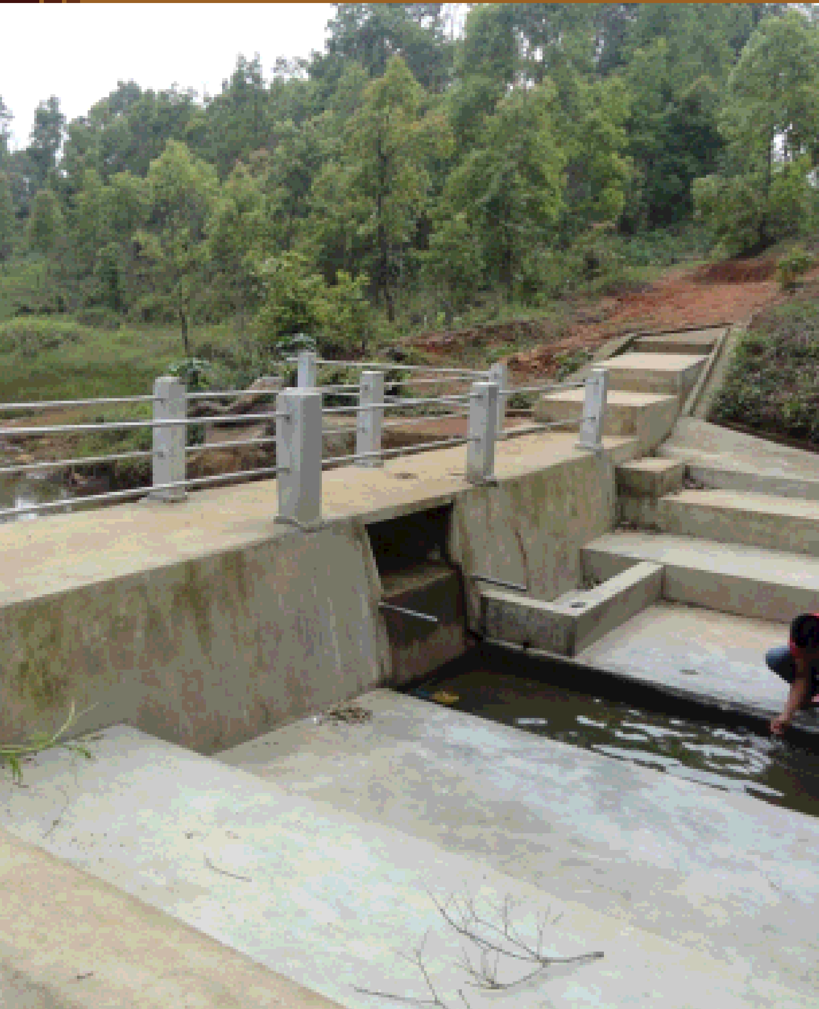
CONSTRUCTION OF WASHING PLATFORM AT POMDKHAR VEC, UMDEIN AEC, MAWSHYNRUT C&RD BLOCK, WEST KHASI HILLS DISTRICT
