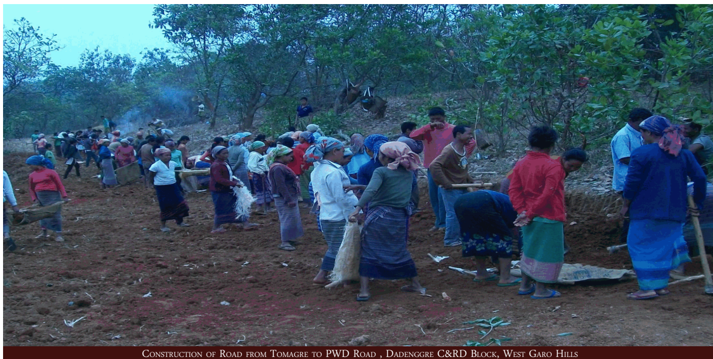
CONSTRUCTION OF ROAD FROM TOMAGRE TO PWD ROAD , DADENGGRE C&RD BLOCK, WEST GARO HILLS
