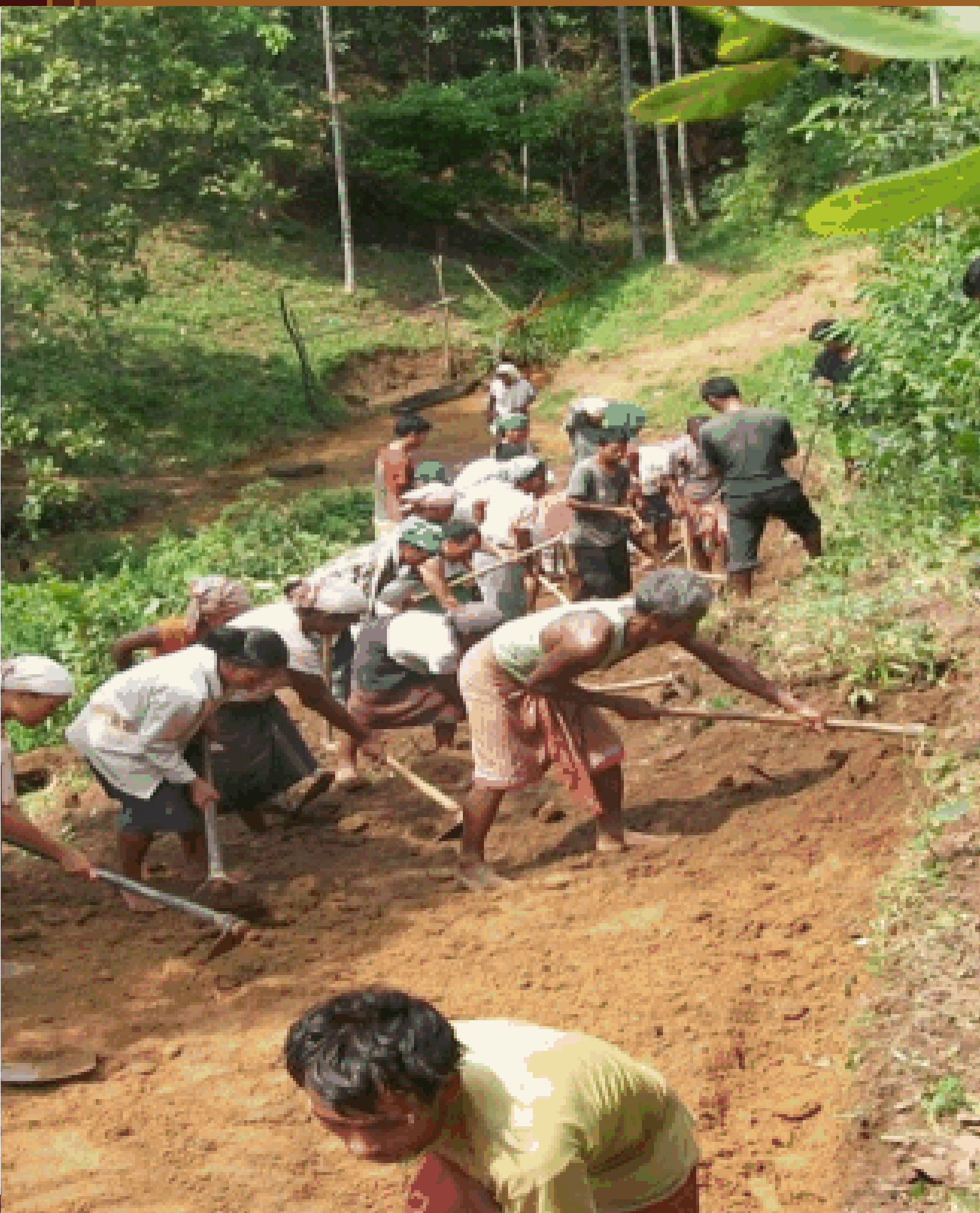
CONSTRUCTION OF ROAD FROM RANGMAI SONGITAL TO RENGQUAGRE, BAGHMARA C&RD BLOCK, SOUTH GARO HILLS DISTRICT
