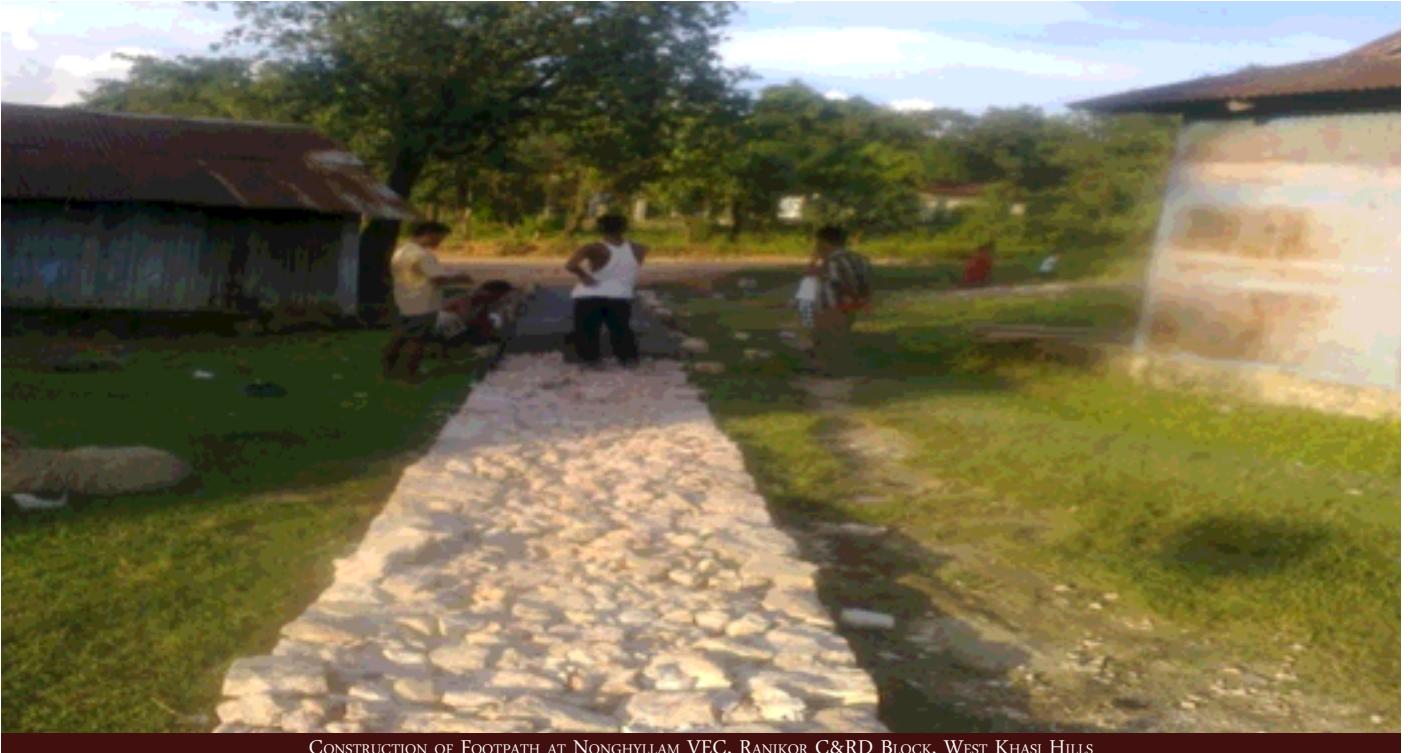
CONSTRUCTION OF FOOTPATH AT NONGHYLLAM VEC, RANIKOR C&RD BLOCK, WEST KHASI HILLS
