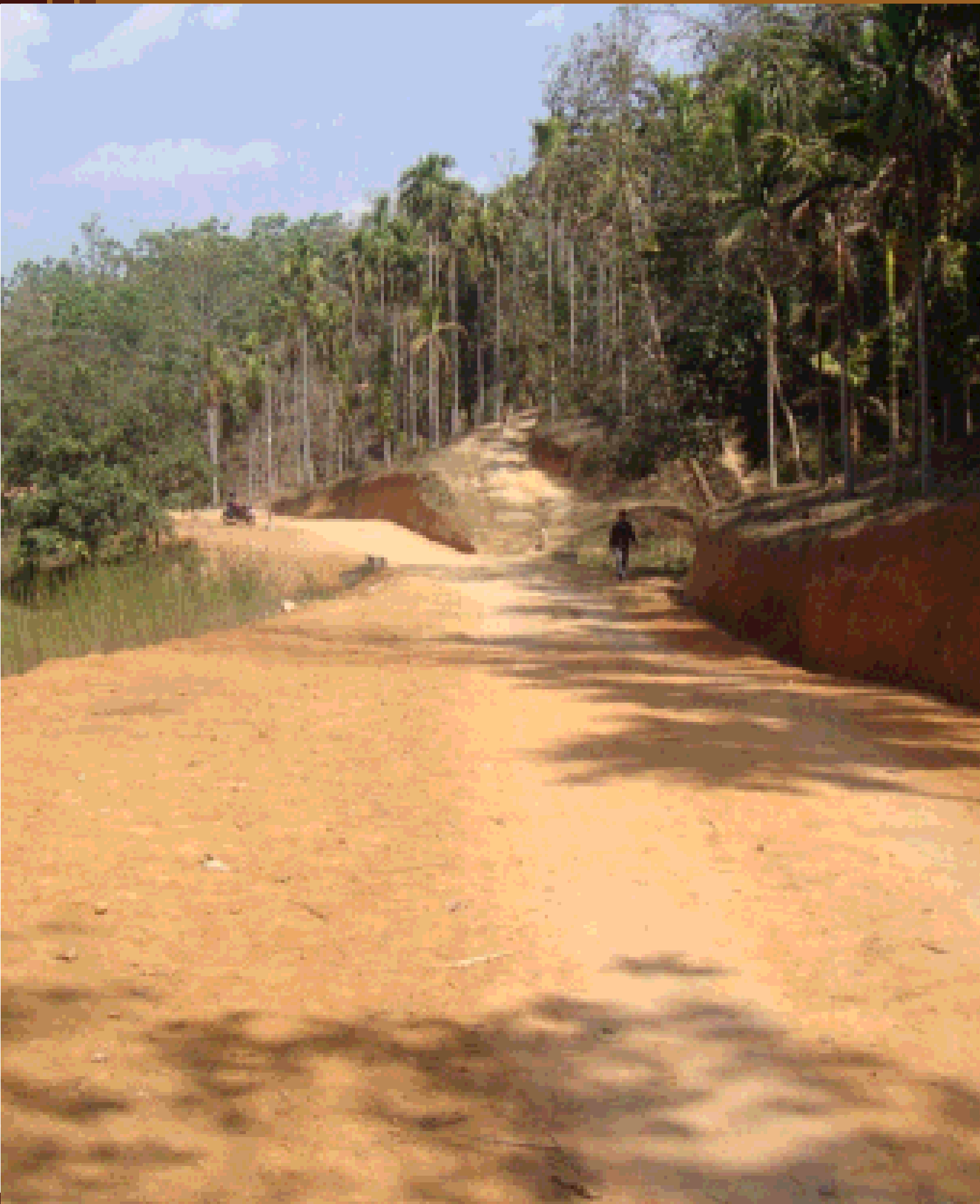
CONSTRUCTION OF ROAD FROM A'SIMGRE TO REBUGRE, DADENGGRE C & RD BLOCK, WEST GARO HILLS DISTRICT
