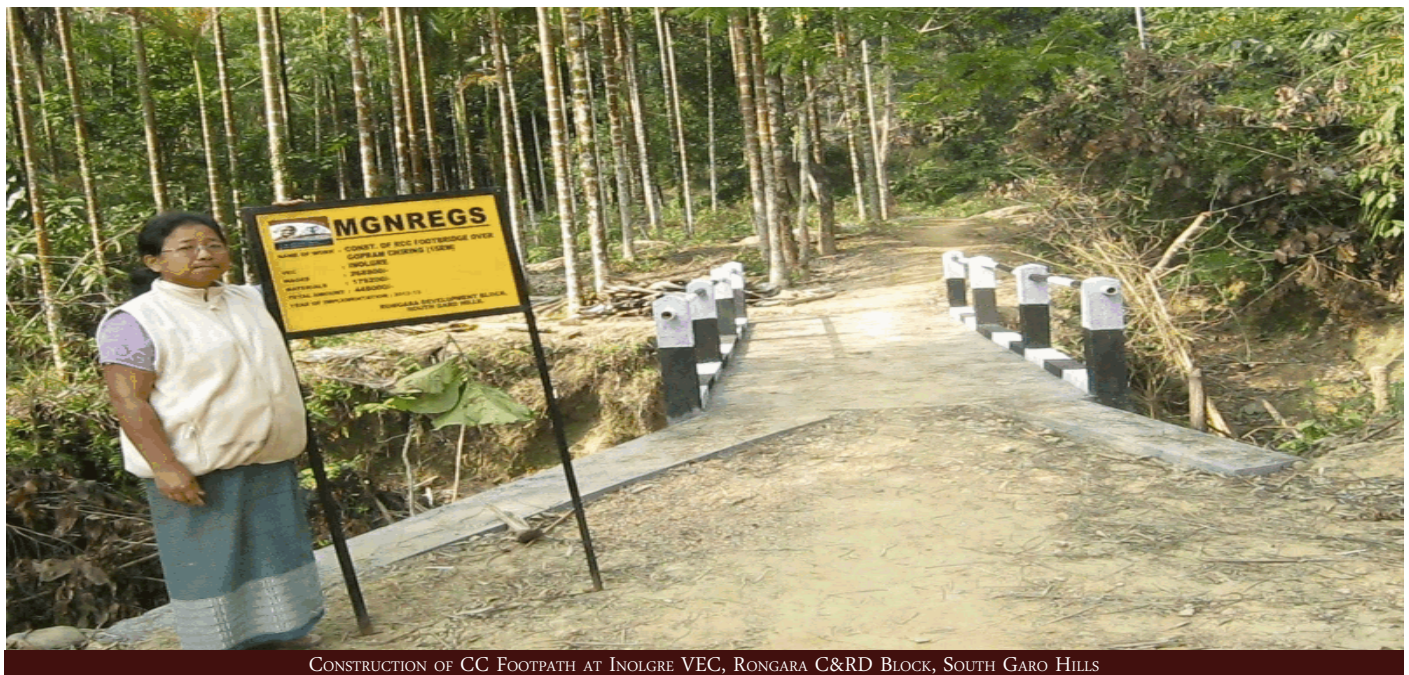
CONSTRUCTION OF CC FOOTPATH AT INOLGRE VEC, RONGARA C&RD BLOCK, SOUTH GARO HILLS
