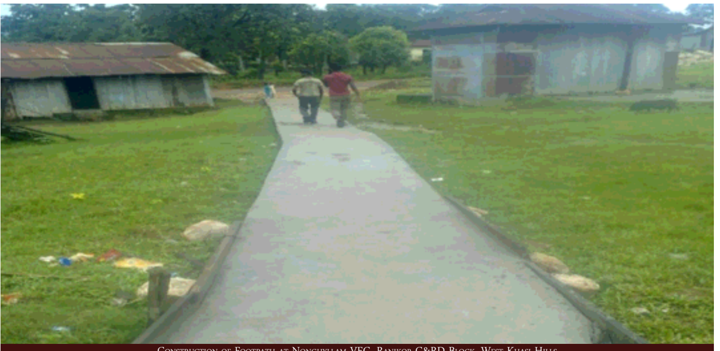
CONSTRUCTION OF FOOTPATH AT NONGHYLLAM VEC, RANIKOR C&RD BLOCK, WEST KHASI HILLS
