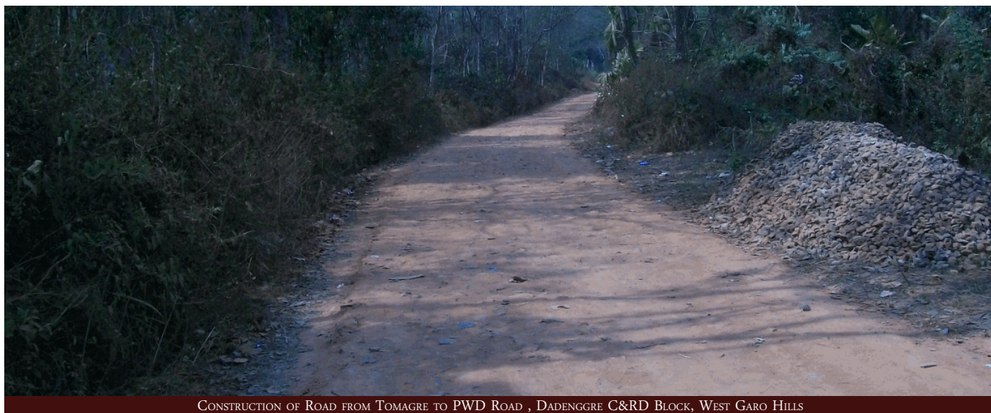
CONSTRUCTION OF ROAD FROM TOMAGRE TO PWD ROAD , DADENGGRE C&RD BLOCK, WEST GARO HILLS
