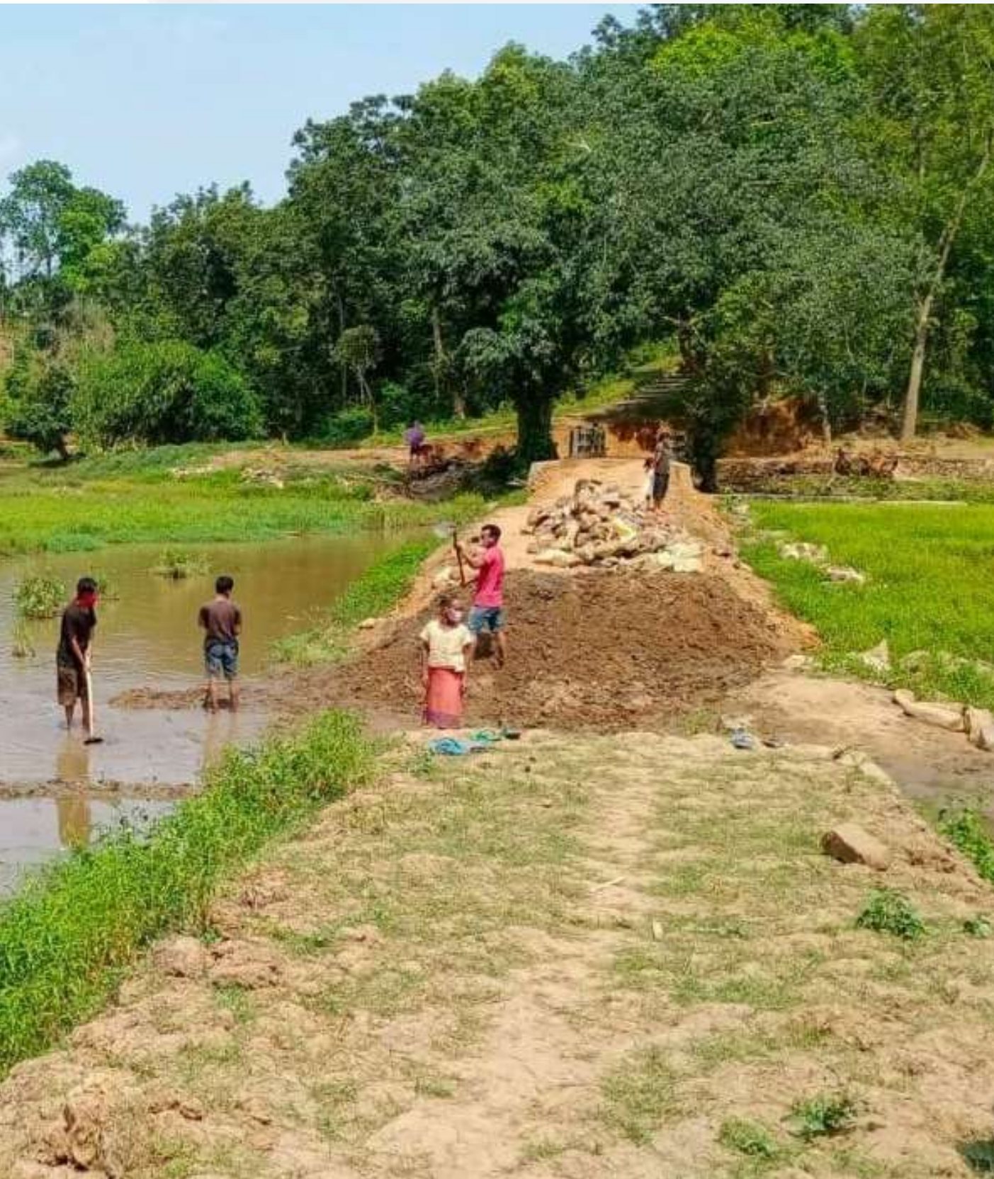
Picture: Construction of Earthen embankment works at Tasek Lake under Songsak C&RD Block, East Garo Hills District
