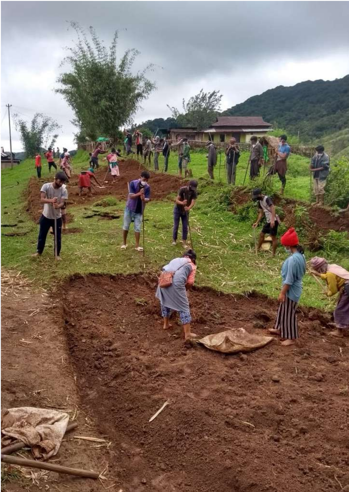
Picture: Construction of Approach Road at Mawroh VEC, Mawthadraishan C&RD Block, West Khasi Hills District
