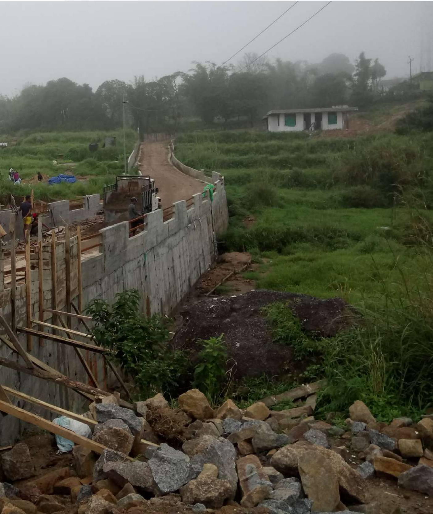
Picture: Construction of Footpath at Nonglang VEC, Mawkyrwat C&RD Block, South West Khasi Hills District
