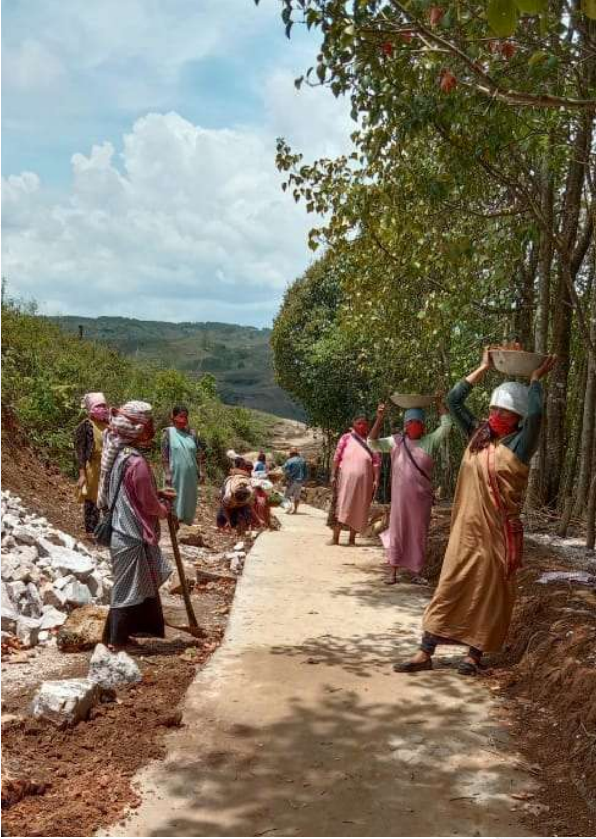
Picture: Construction of Footpath at Mukhatalong VEC, Khliehriat C&RD Block, East Jaintia Hills District
