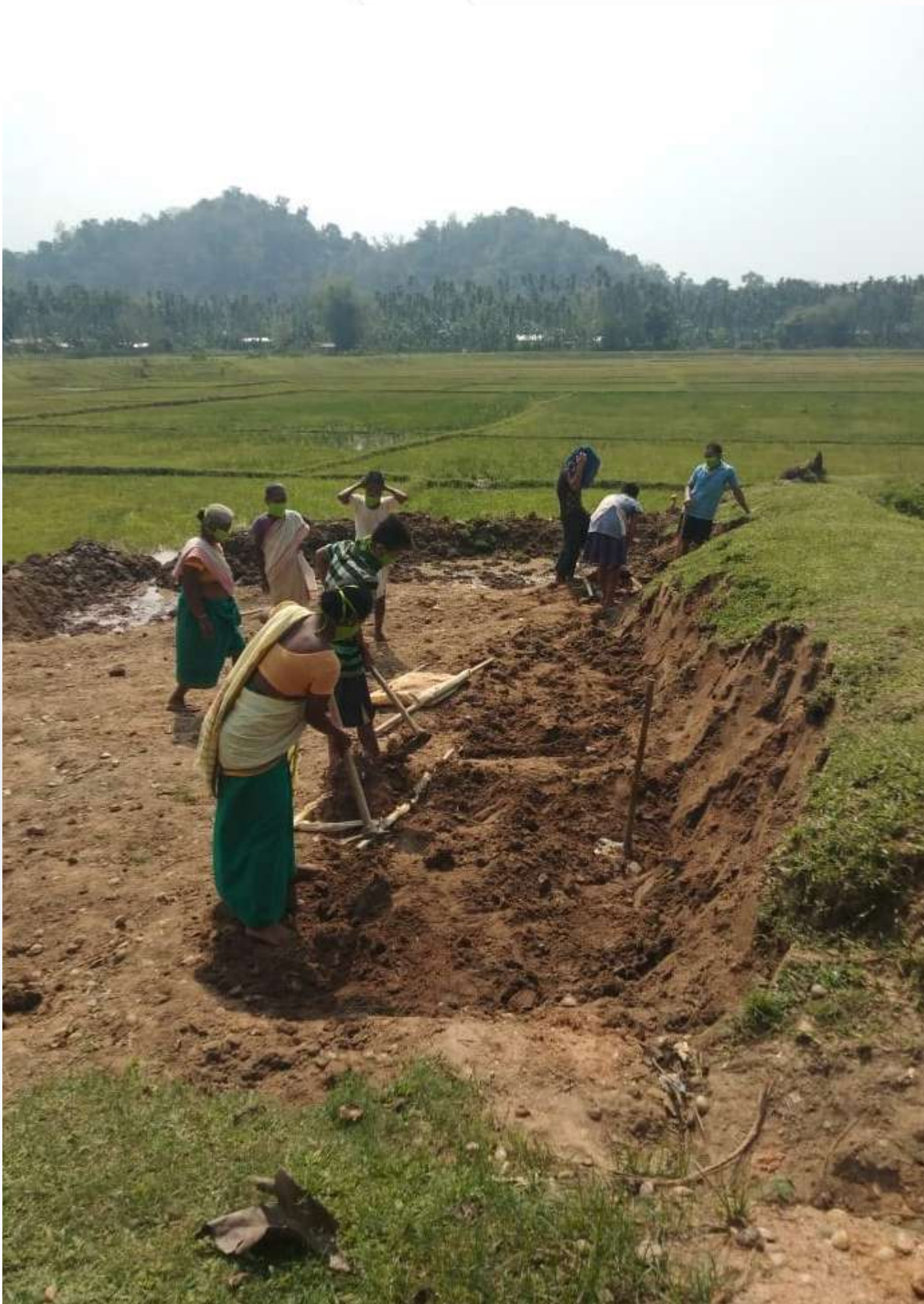
Picture: Construction of water conservation pond at Akhoijira VEC, Jirang C&RD Block, Ri Bhoi District
