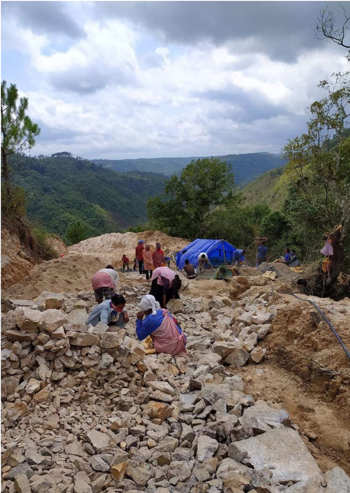
Picture: Job Card Holders constructed a CC Road at Tuberkmaishnong VEC, Khliehriat Block, East Jaintia Hills District
