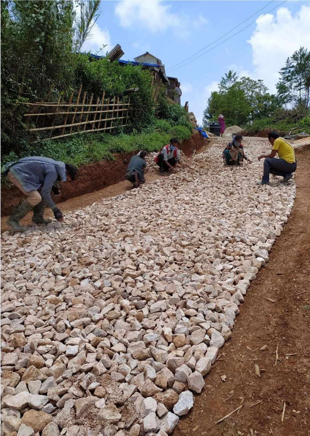
Picture: Job Card Holders constructed a CC Road at Tymphakasu VEC, Saipung Block, East Jaintia Hills District
