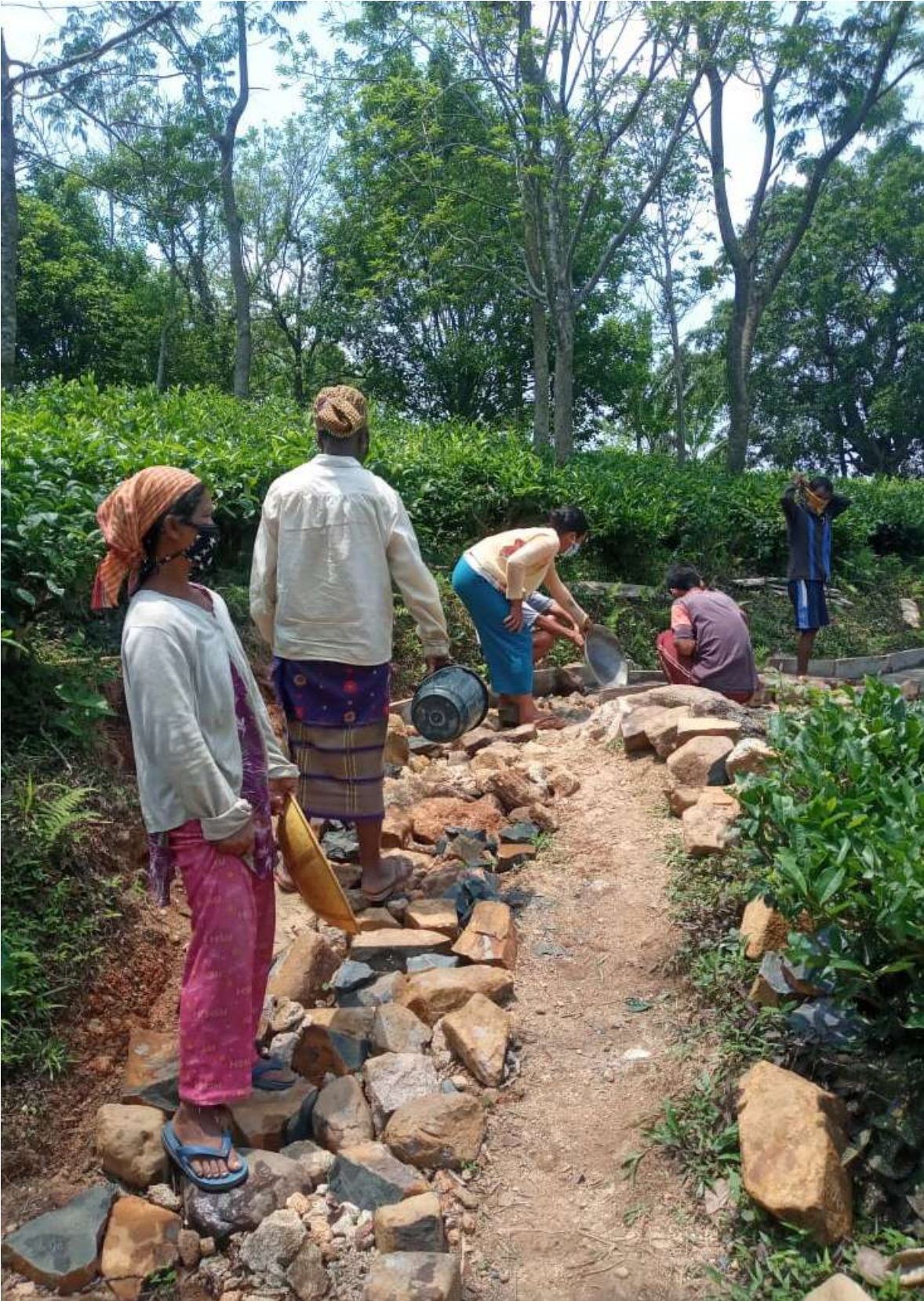
Picture: Construction of Footpath, Aguragre VEC, Rongram C&RD Block, West Garo Hills District
